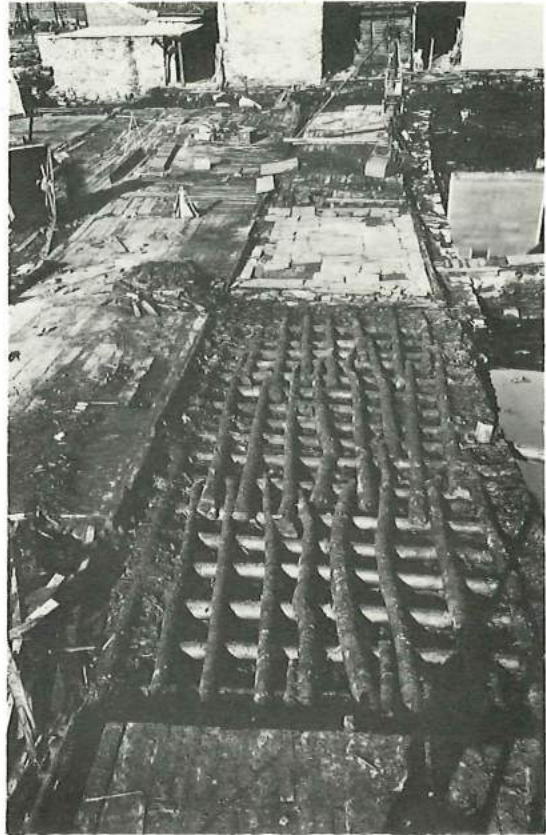
Fig 6 Situation following 1955 fire. Large parts of the wooden floors in the lower storey were intact. In most cases and especially at deeper levels, the fire caused extensive damage deep down into the foundations
